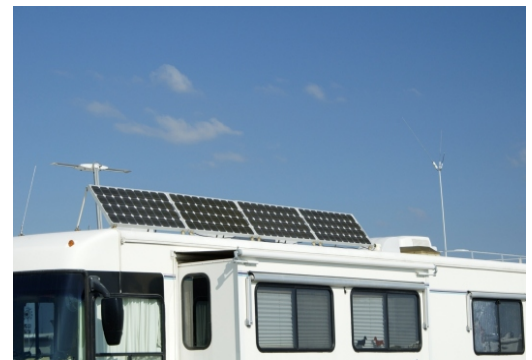
A PV array installed upon a caravan
